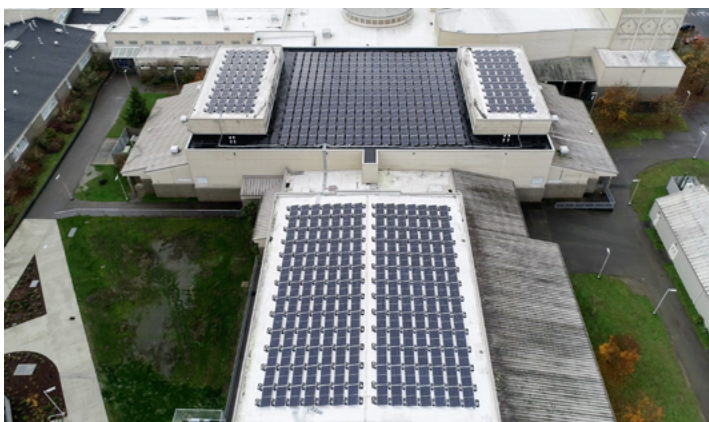
More than 500 solar panels were installed on the roof of Olympia High School as part of Puget Sound Energy's first Community Solar project.
